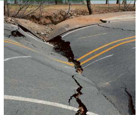
Road after earthquake
